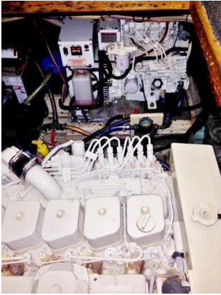
Engine & Generator Beneath Pilothouse Sole
